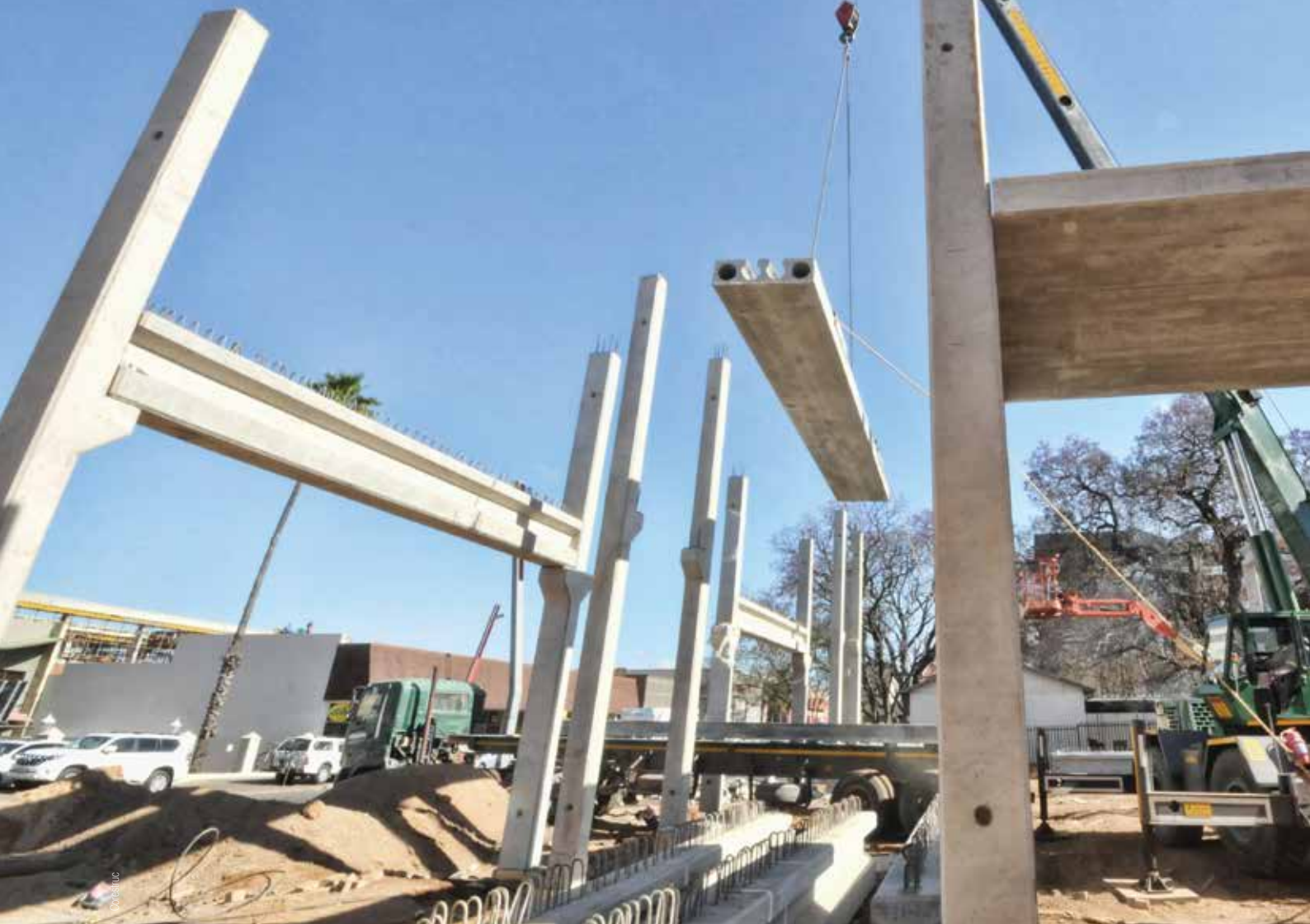
Smaller skilled teams are tasked with the installation of the precast concrete structure.
