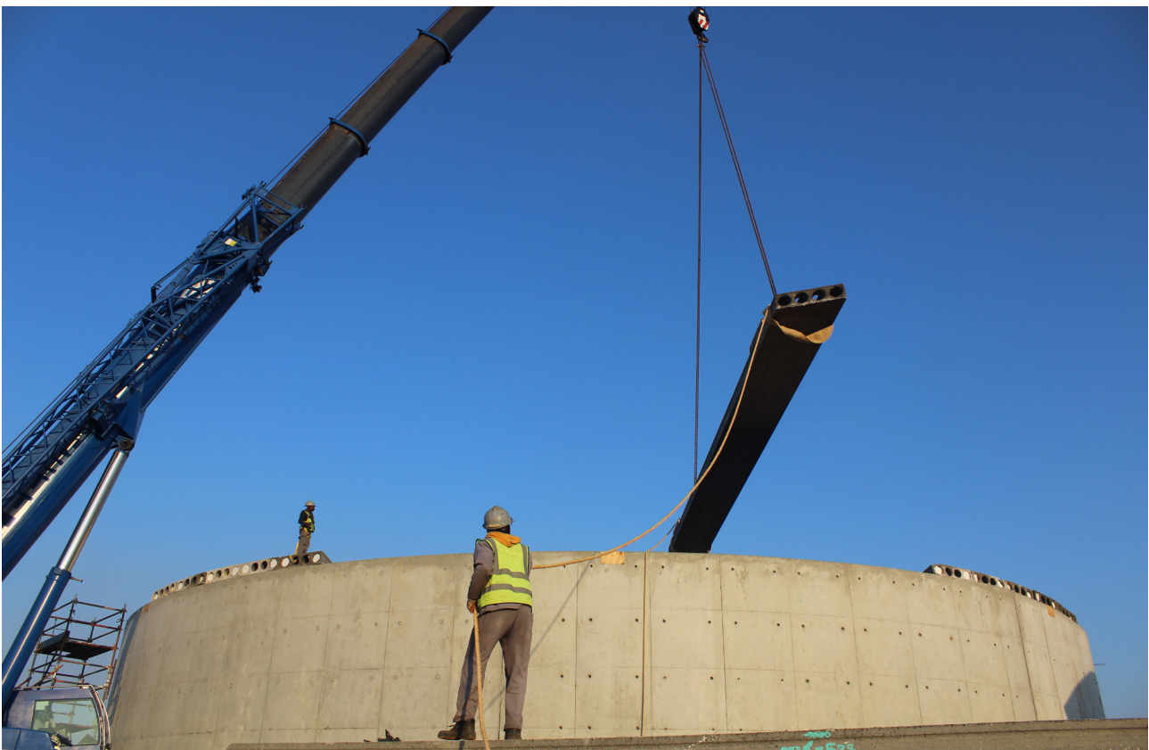
The hollow-core slabs are supported directly by the load-bearing walls. This includes a wall inside the structure that divides it into two separate water retaining compartments.
